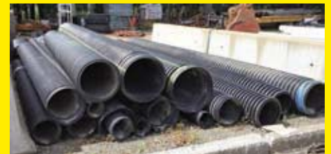
QTY OF LARGE DIAMETER PLASTIC PIPE
